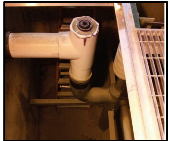
Influent plumbing connected to cell wall and feed chamber inlet pipe stub.
