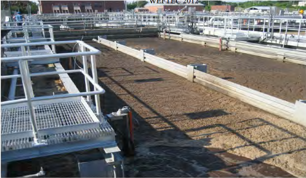
Figure 8 – View of Post Anoxic Zone Cell 5 & 6; Fiberglass Baffle Walls
