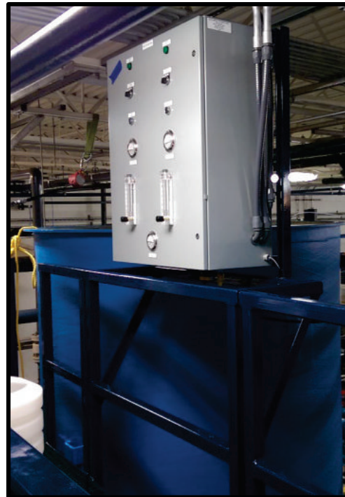
Handrail mounted air panel
