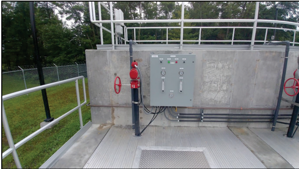
Example of air panel installed.
