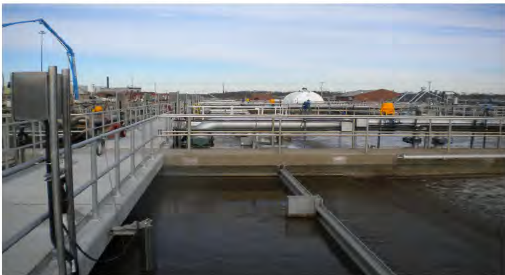
Figure 7 –View of Quiescent Pre-Anoxic Zone in a Tank; Mixer Mast in Foreground
