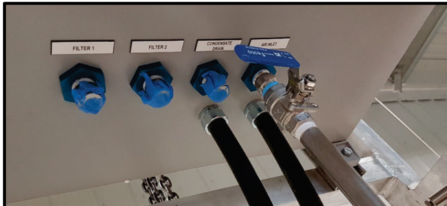
Air control panel connections: power, air supply, and filter air.
