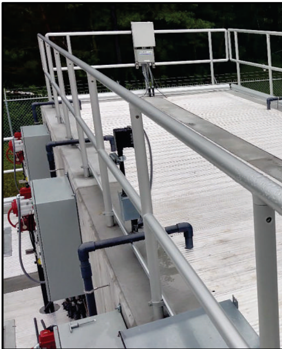
Venting installed on concrete cell, draining to influent trough.
