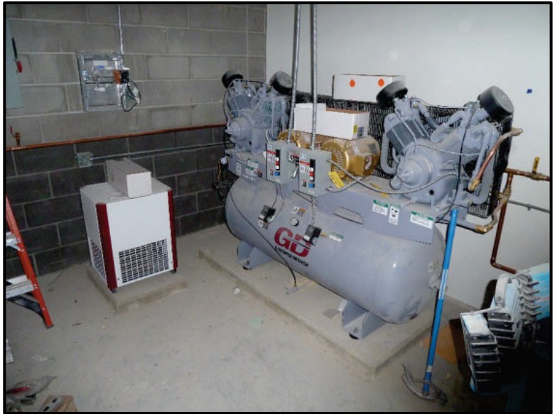
Example of an air compressor on site
