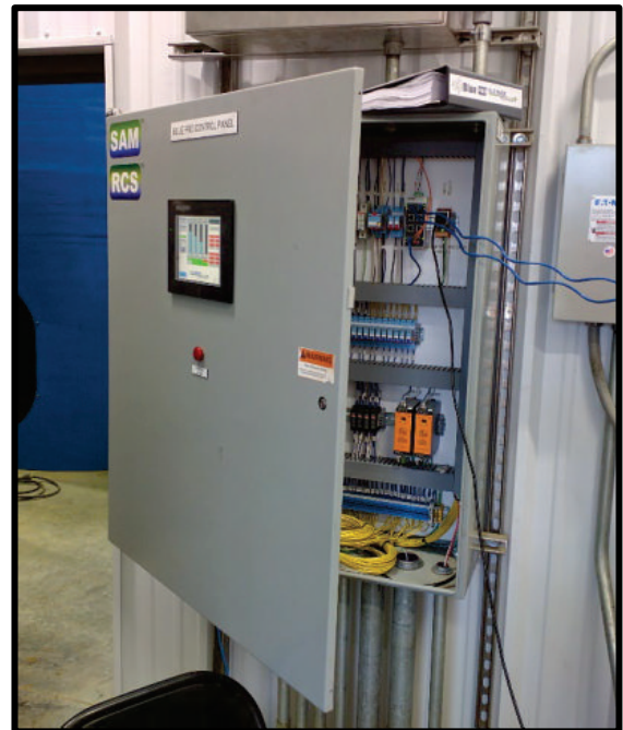
Wall mounted filter control panel during system installation.
