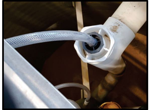
Venting hose connected to influent plumbing assembly and feed chamber.
